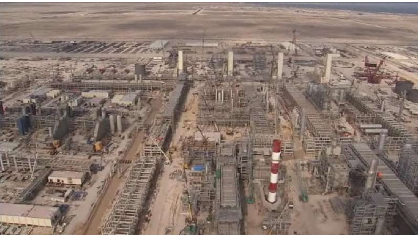
Pearl Shell GTL site at Ras Laffan
