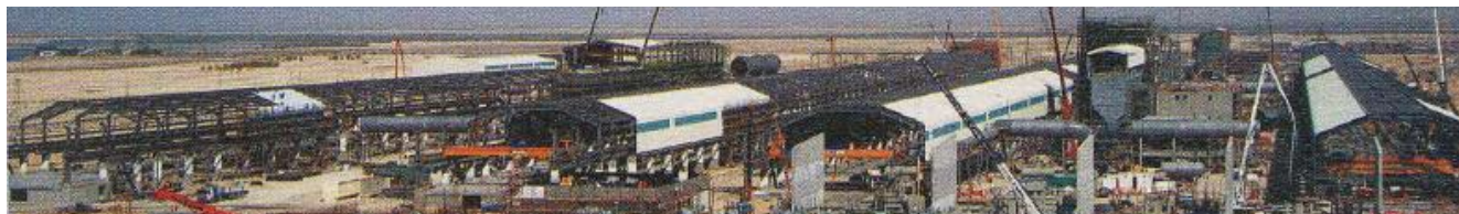
Inter-tie transformer equipment in the Energy area The first cathode sealing, on 29 April 2009
