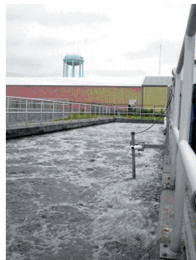
Endress+Hauser COS 41 sensor mounted in aeration tank with pendulum holder which provides easy access to wipe sensor membrane
